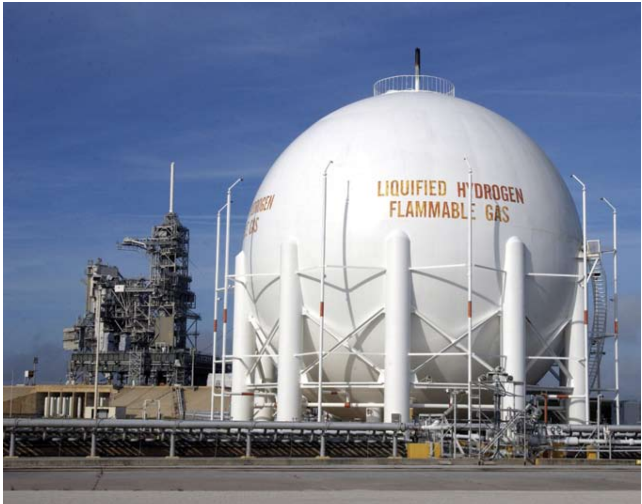
A large round tank that is actually a high vacuum bottle stores the supercold liquid hydrogen at the launch pad. A similar round vessel holds the liquid oxygen. The liquid propellants flow to the orbiter's main engines.
